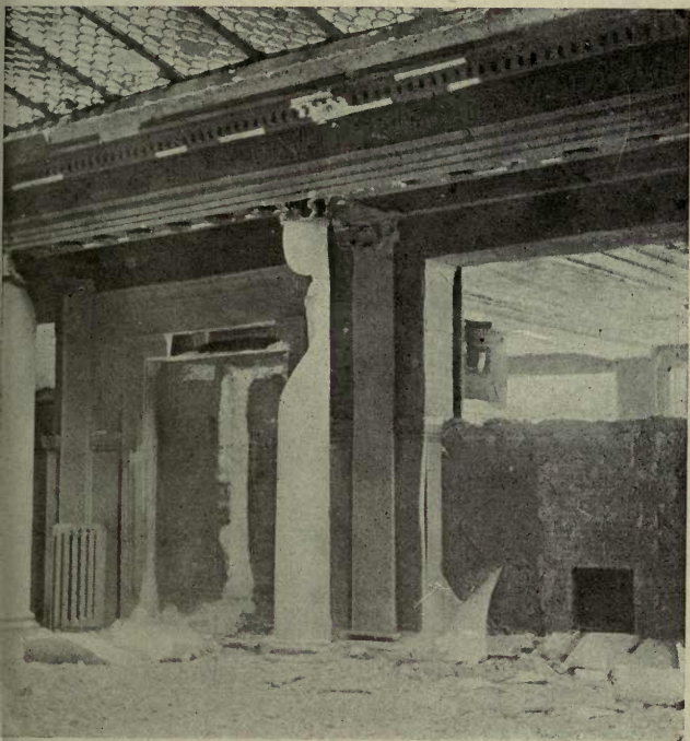
FIG. 36. — Entrance Rotunda of Calvert Building, Baltimore Fire.
